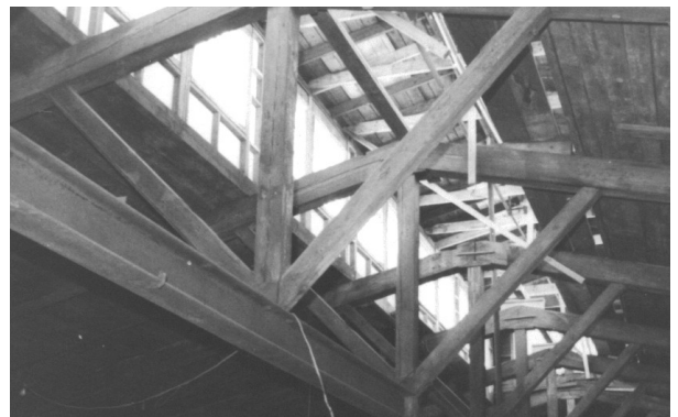
The AAIM clerestory monitor window during renovations in August, 1979. Photo taken by Elizabeth Hartshorn Phillips.
